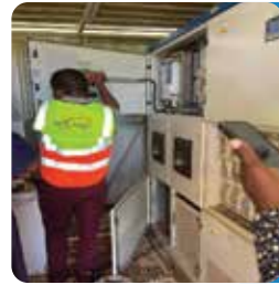
Finding faults at the Main LV Panel of NFRA Sumbawanga
