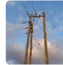
Line of Three members Poles on heavy angle at Kasinde village
