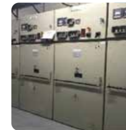
Main MV Switchgear for CCBRT hospital project
