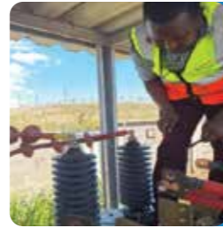
Testing of transformer at the NFRA Kanondo Sumbawanga
